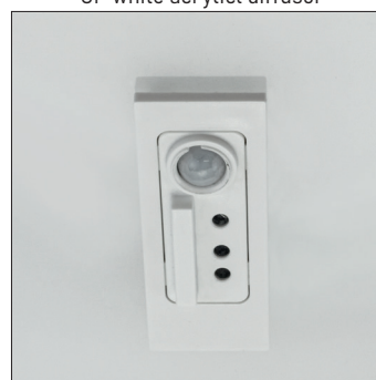
XC daylight&occ sensor
